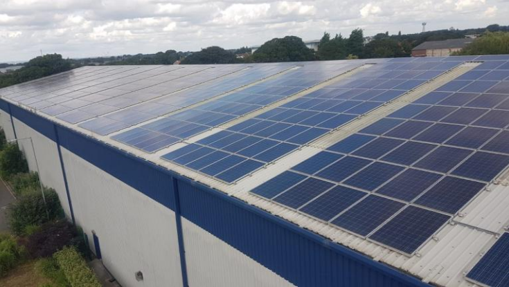
Solar Panels on the roof of Bio-D's HQ.
